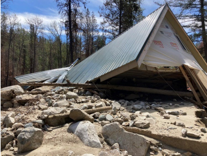
Figure 3.c.6. The impacts of post-fire debris flow near Conconully in July 2022. (Source: Eli Loftis, Okanogan CD, 2022)
