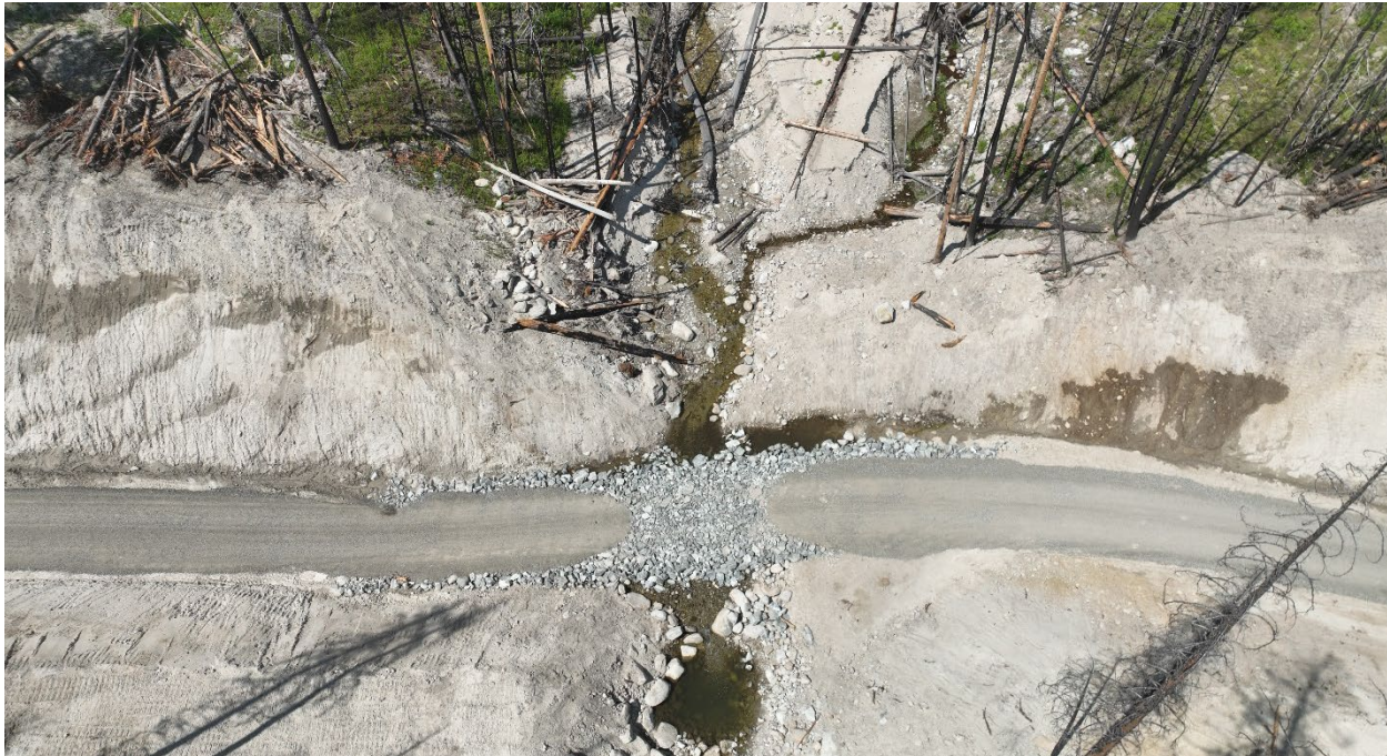
Figure 1.b.10. Debris flows, floods and other post-fire hazards can require significant effort to mitigate and possibly obstruct future firefighting efforts. This crossing was constructed by the Tonasket Ranger District in the aftermath of repeated blowouts of Lightning Creek in the Okanogan Highlands after the 2021 Walker Creek Fire. (Source: Mike Baden, WSCC, 2024)
